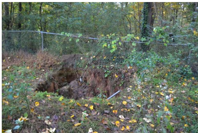
Figure 3-11. Stormwater Drainage Issue Contributing TSS to the Study Area
