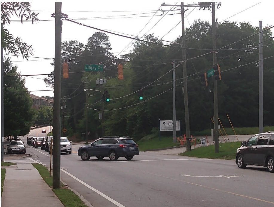
GREEN ARROW DOES NOT TURN ON AT THE ELLIJAY DRIVE INTERSECTION FOR VEHICLES IN THE LEFT-TURN LANE
