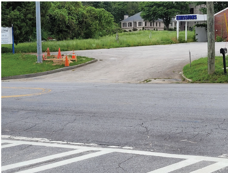
NO SIDEWALK OR CURB RAMPS ON THE NORTH SIDE OF DRESDEN DRIVE BETWEEN PARKSIDE DRIVE AND CALDWELL ROAD
