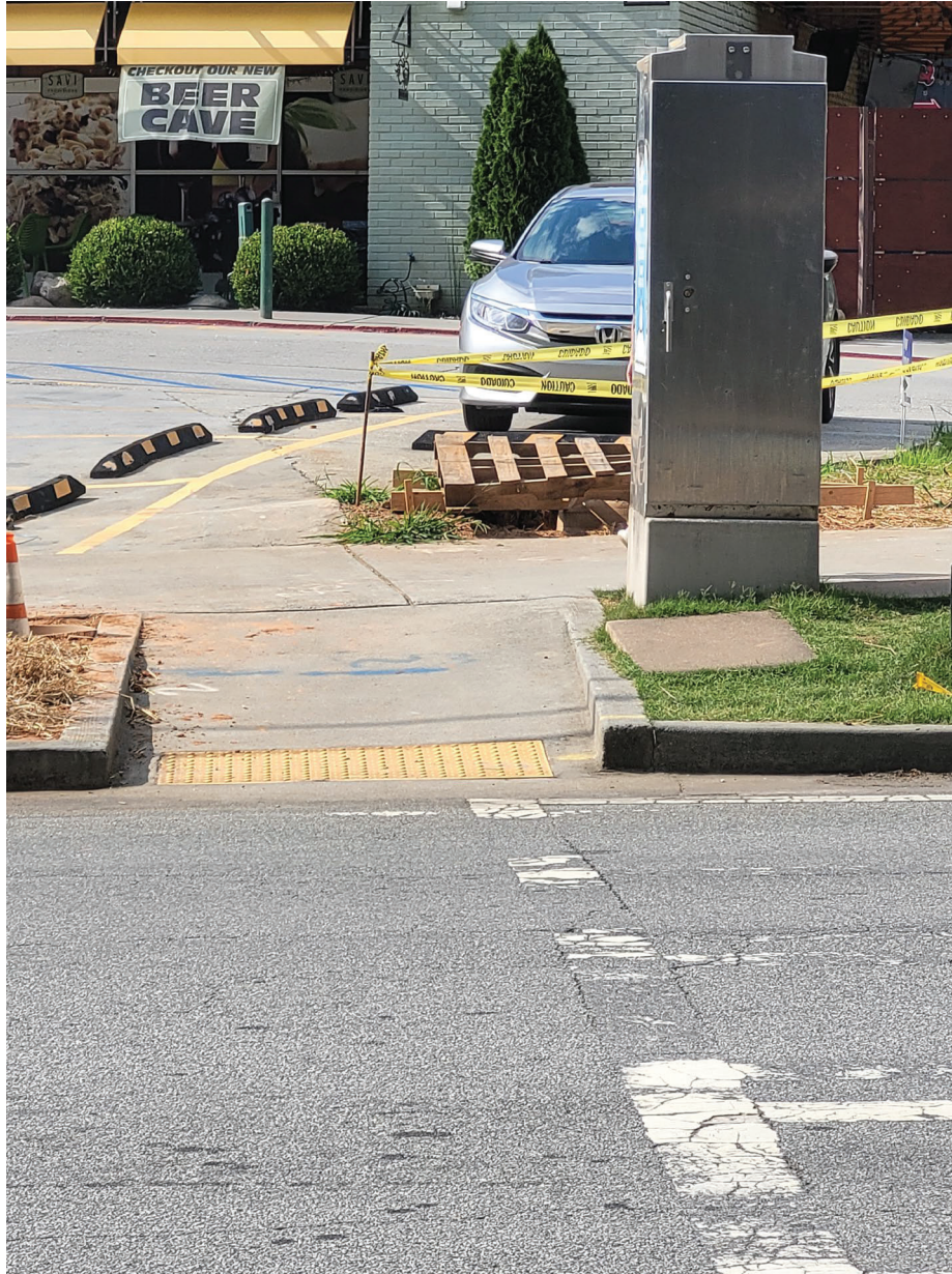
PAVEMENT MARKINGS AND CURB RAMP ON THE WEST LEG OF THE CALDWELL ROAD INTERSECTION DO NOT ALIGN
