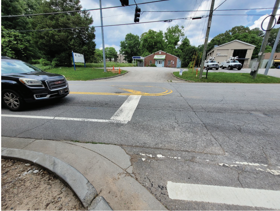
NO CURB RAMPS OR CROSSINGS AT THE WEST LEG OF THE INTERSECTION
