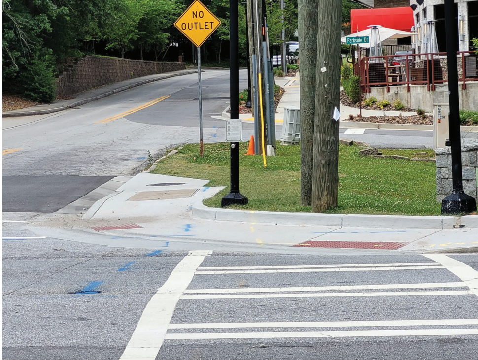
SIDEWALK GAP BETWEEN THE INTERSECTION AND BUSINESS NORTH OF PARKSIDE DRIVE ALONG APPLE VALLEY ROAD
