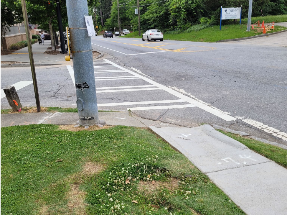
NARROW CURB RAMP ON THE SOUTHEAST CORNER OF THE ELLIJAY DRIVE INTERSECTION
