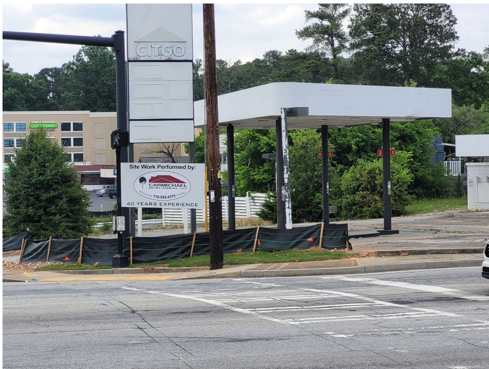
SITE DEVELOPMENT WORK UNDERWAY AT FORMER GAS STATION ON THE NORTHEAST CORNER OF THE INTERSECTION
