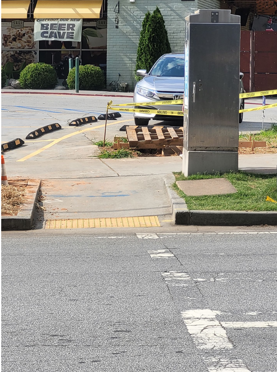
PAVEMENT MARKINGS AND CURB RAMP ON THE WEST LEG OF THE CALDWELL ROAD INTERSECTION DO NOT ALIGN
