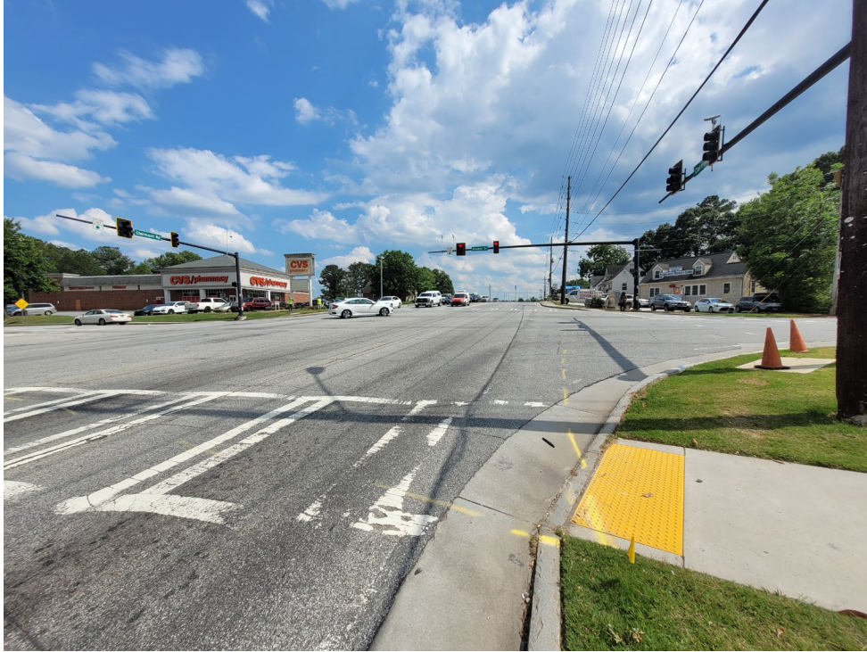
WORN CROSSWALK PAVEMENT MARKINGS IN THE NORTH LEG OF THE INTERSECTION
