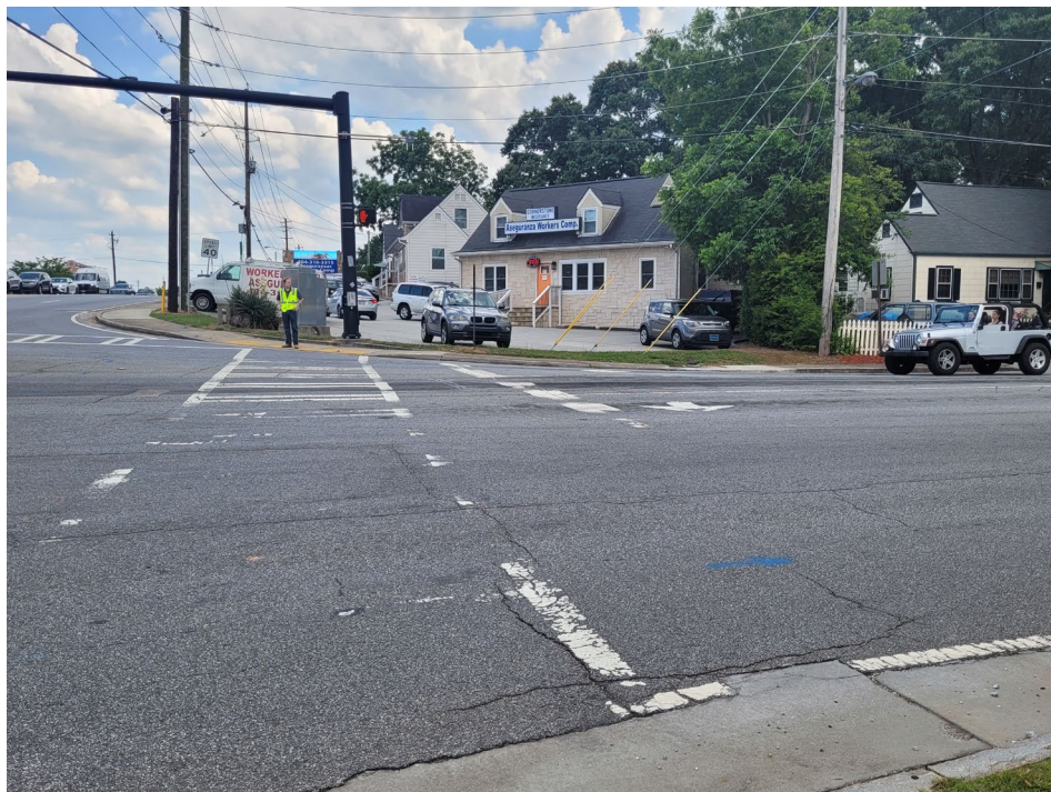
WORN CROSSWALK MARKINGS IN THE WEST LEG OF THE INTERSECTION
