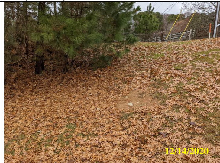
23. High traffic area at right side of downstream dam face showing erosion and missing grass
