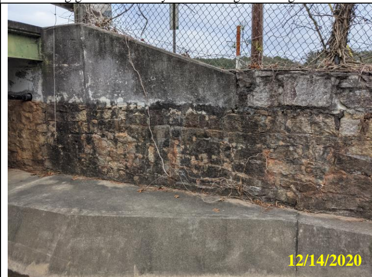
39. Remains of vines and vegetations on masonry wall downstream of bridge crossing
