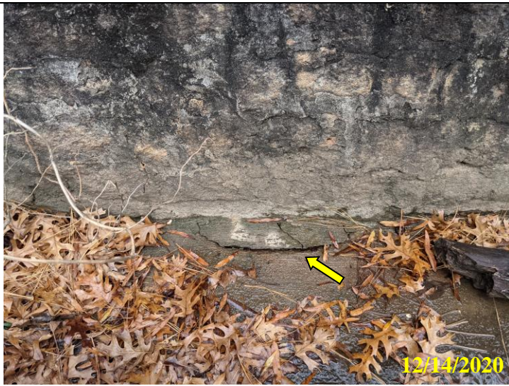
31. Concrete spillway cracking and uplift at masonry wall joint
