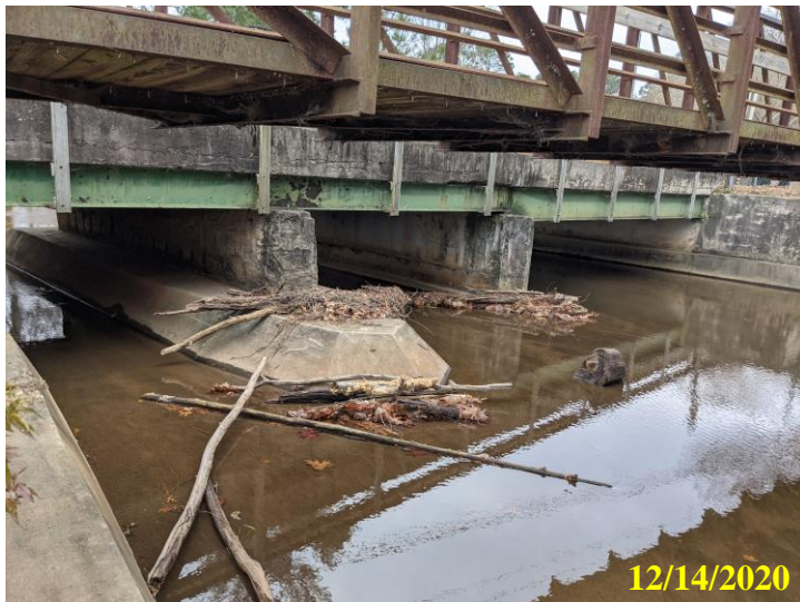
29. Small amount of woody debris accumulation in the upstream section of concrete spillway
