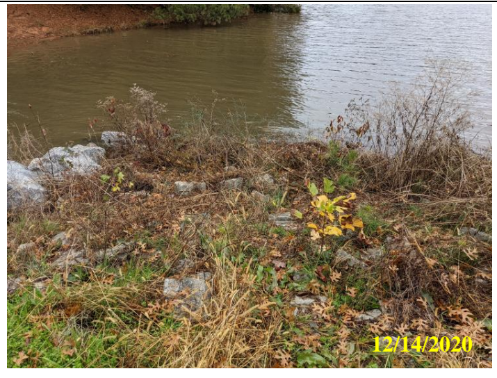
14. Sparse riprap near pedestrian walkway
