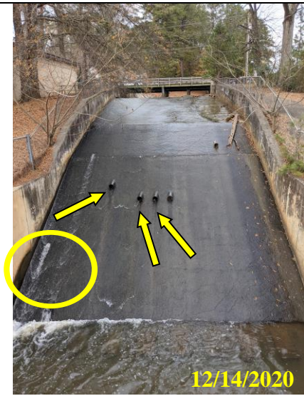
43. Spillway face above plunge pool showing locations of toe drains with missing animal guards, yellow circle shows general area of suspected void behind spillway face
