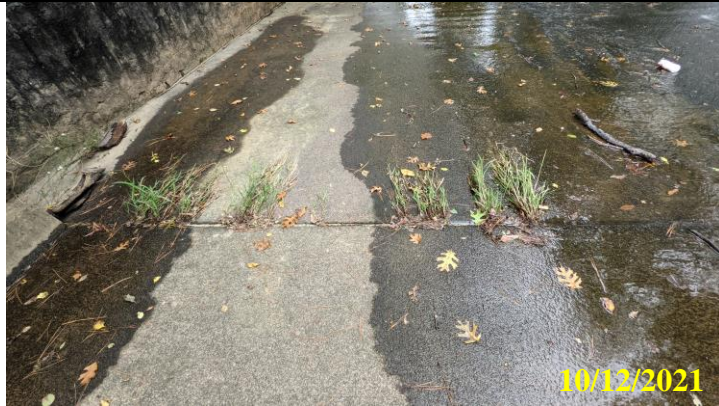
35. Grass growing between slabs in concrete spillway
