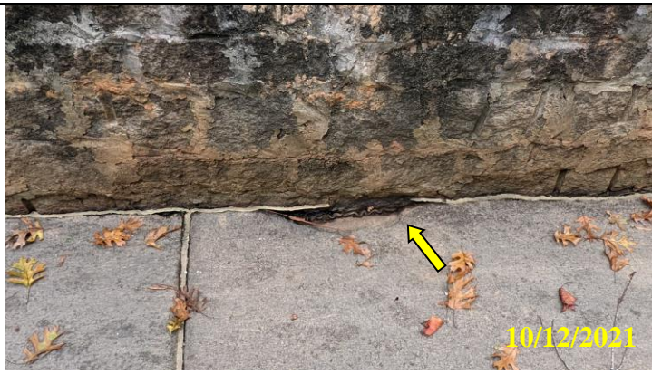
33. Concrete spillway cracking and spalling concrete at masonry wall joint
