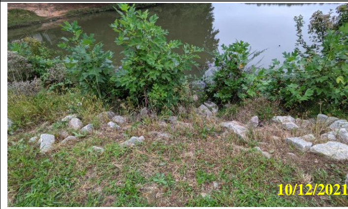
15. Sparse riprap coverage and uneven riprap sizing at right side of upstream dam face
