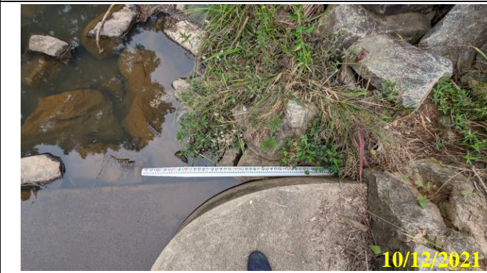
11. Inadequate riprap grading at the left wing wall of the concrete spillway resulting in erosion and undercutting of riprap. See Photo 12 for location of this photo
