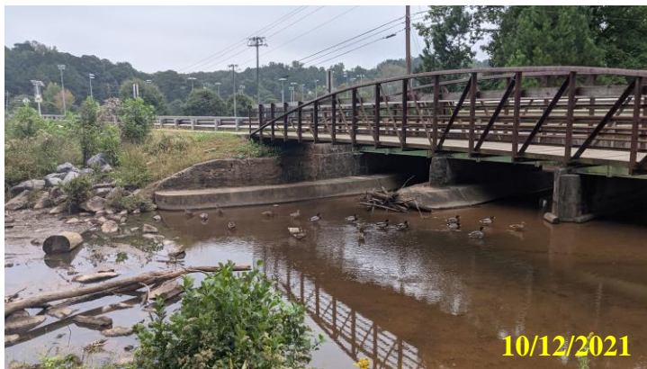
29. Woody debris accumulating in the upstream section of concrete spillway
