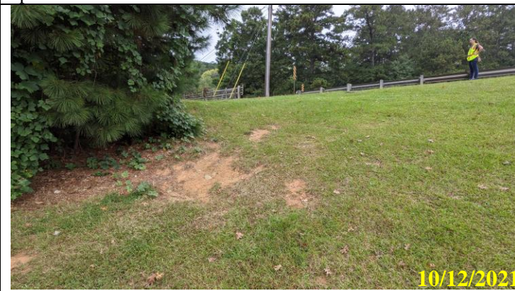
23. Right side of downstream dam face showing erosion and missing grass
