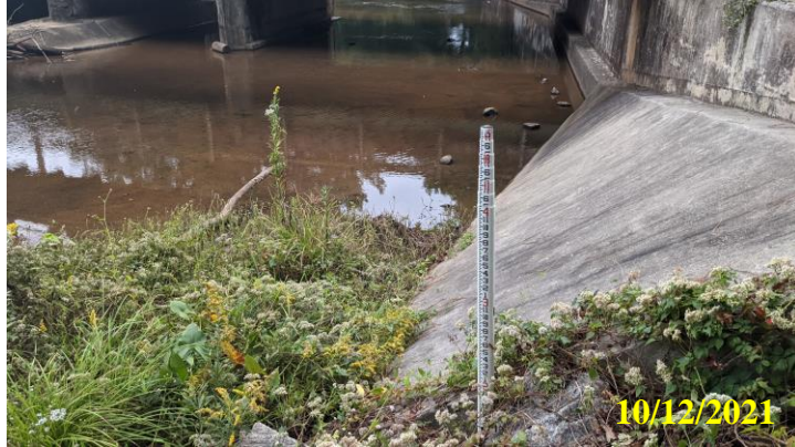
27. View of overgrown vegetation and sparse poorly graded riprap at the right upstream wingwall
