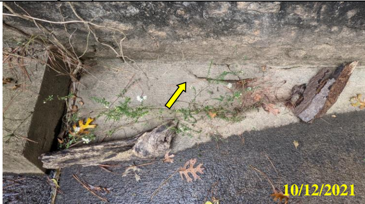
31. Concrete spillway cracking and uplift at masonry wall joint
