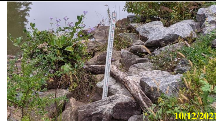
13. Inadequate riprap grading at the left wing wall of the concrete spillway resulting in erosion and undercutting of riprap
