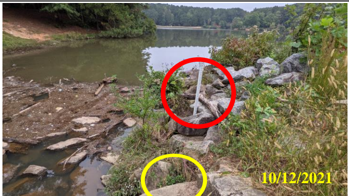
12. Inadequate riprap grading at the left wing wall of the concrete spillway resulting in erosion and undercutting of riprap. Yellow circled area is location of Photo 11 and red circled area is location of Photo 13
