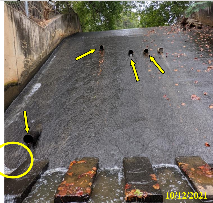
43. Spillway face above plunge pool showing locations of toe drains with missing animal guards. Yellow circle shows general area of suspected void behind spillway face
