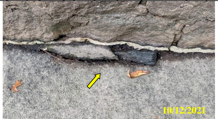
32. Concrete spillway cracking and uplift at masonry wall joint with exposed seal
