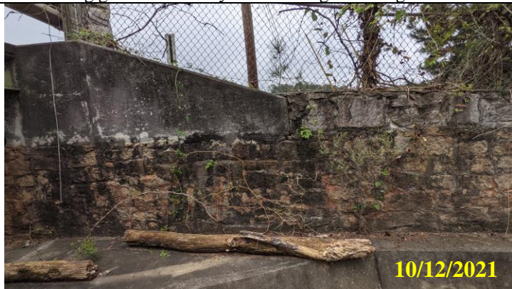
39. Vines and vegetations on masonry wall downstream of bridge crossing
