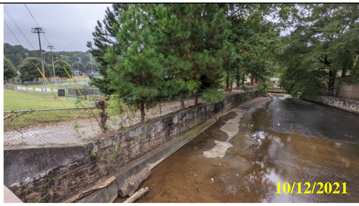
42. Trees at spillway fence
