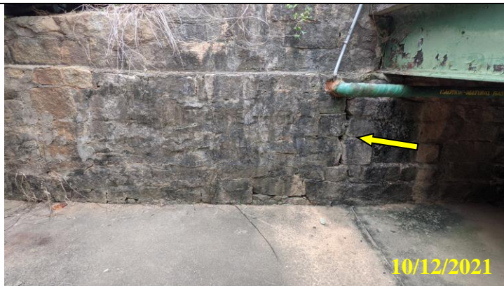
37. Missing grout in masonry wall at bridge crossing
