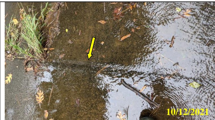
41. Caulk peeling from between spillway slabs downstream of bridge crossing
