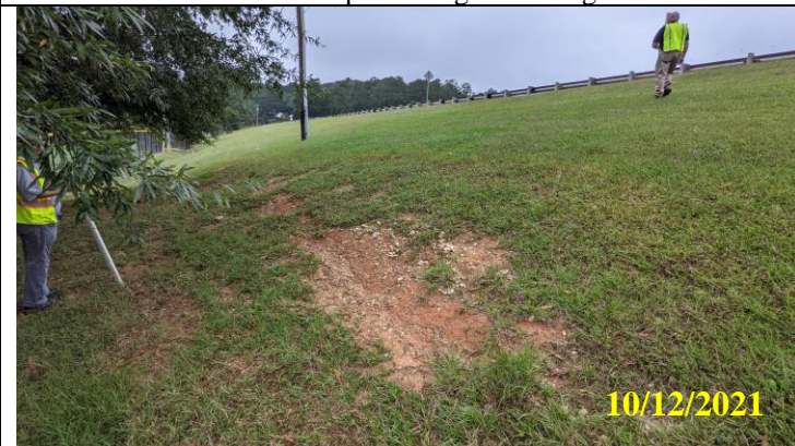
19. Patches of missing grass on downstream dam face
