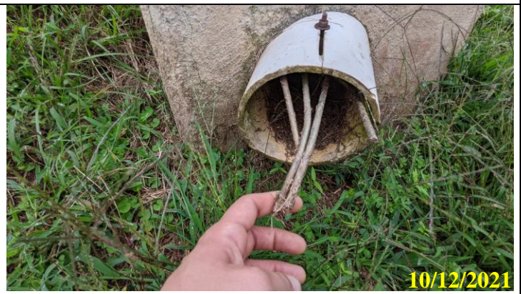
24. Toe drain at center of downstream dam face showing damaged animal guard
