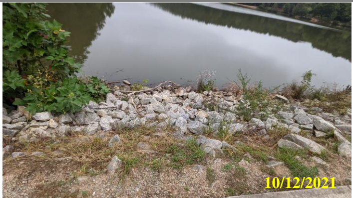
14. Sparse riprap near pedestrian walkway
