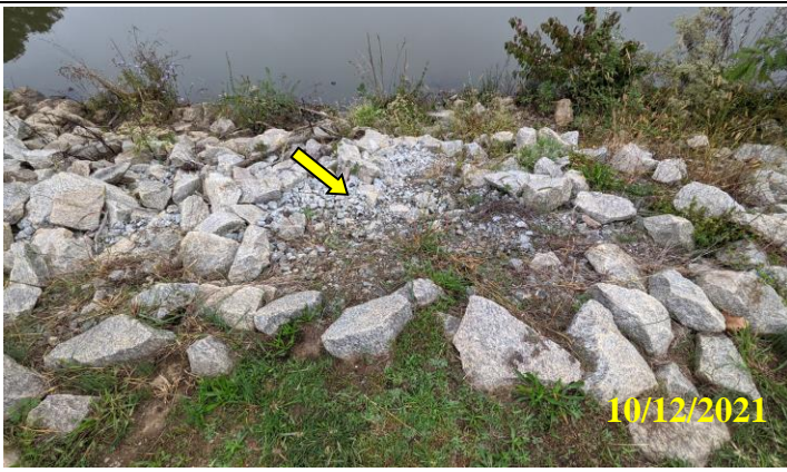
16. Pedestrian pathway showing sparse riprap near principal spillway riser
