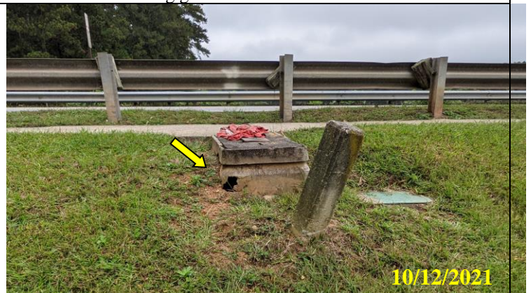
22. Damaged utility box on downstream face of dam
