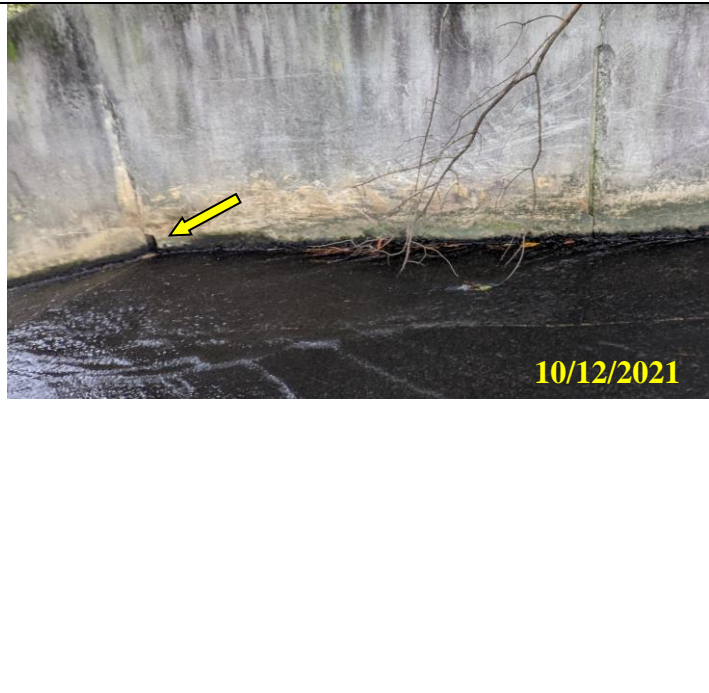
44. Cracked and missing concrete at top left of plunge pool face
