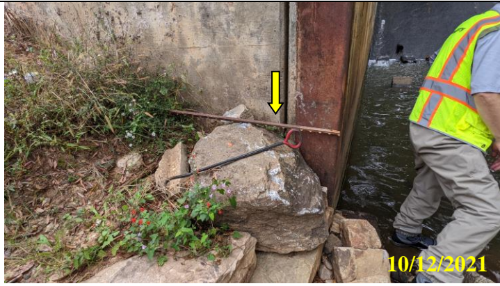
25. Toe drain at right side of plunge pool obscured by newly placed riprap
