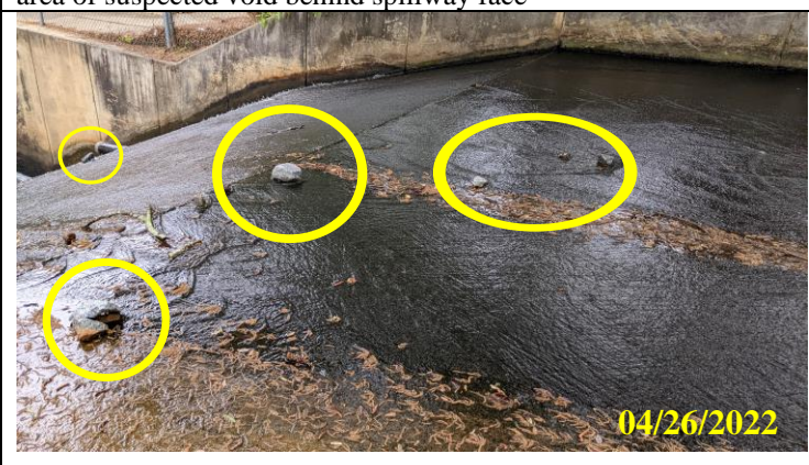
45. Riprap thrown into spillway
