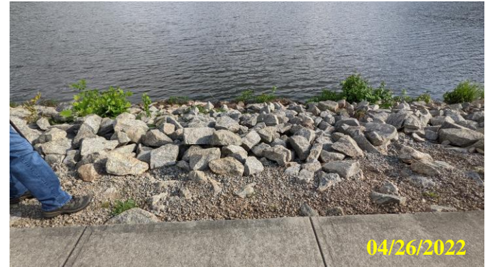
14. Sparse riprap near pedestrian walkway
