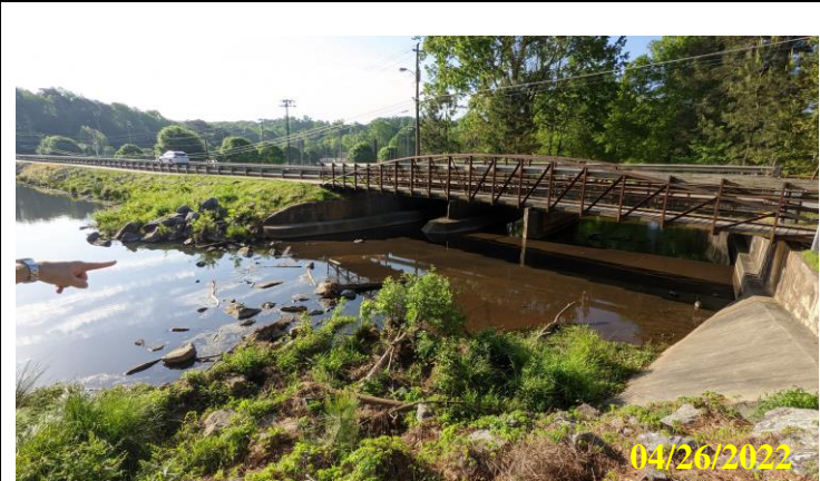
29. Small amounts of woody debris accumulating in the upstream section of concrete spillway
