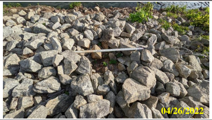
10. View of disturbed riprap around cut back woody vegetation on upstream face of the dam
