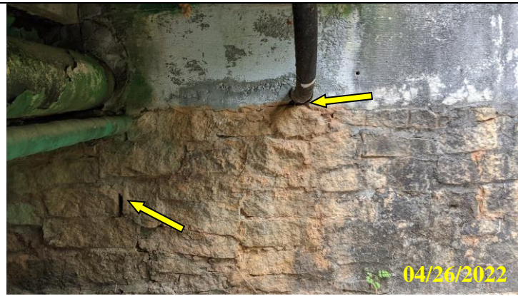
38. Missing grout in masonry wall at bridge crossing
