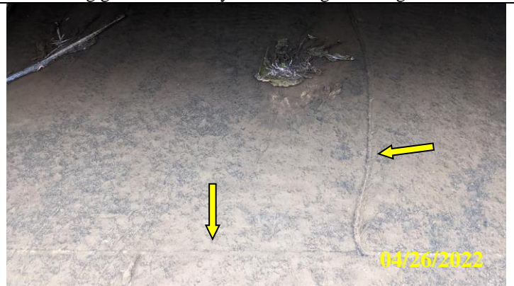
40. Caulking peeling from between spillway slabs at upstream edge of bridge crossing, 6 inch void between slabs
