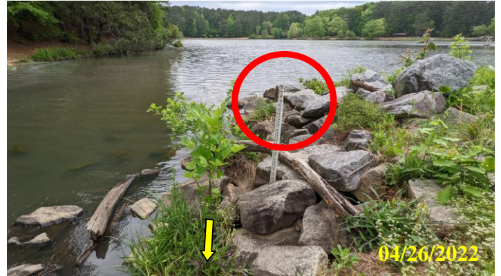
12. Inadequate riprap grading at the left wing wall of the concrete spillway resulting in erosion and undercutting of riprap. Red circled area is location of Photo 13, yellow arrow pointing towards location of Photo 11
