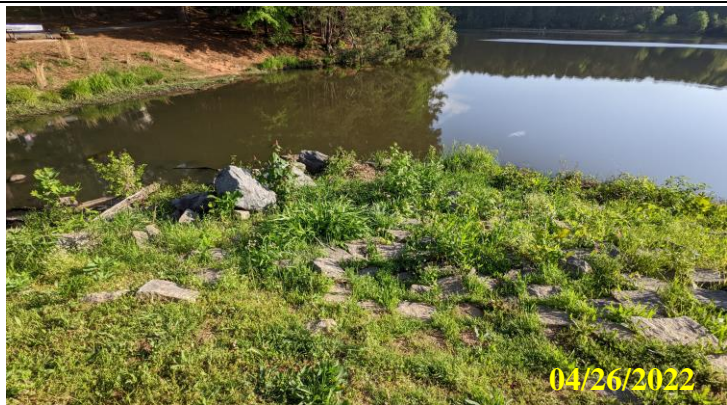
15. Very sparse riprap coverage at right side of upstream dam face
