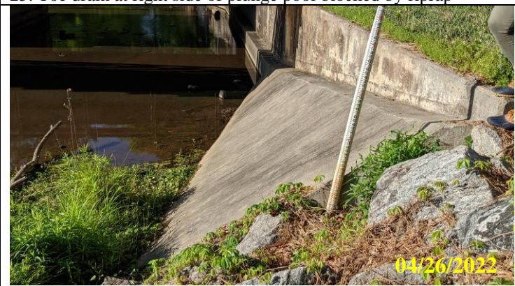
27. View of overgrown vegetation and sparse poorly graded riprap at the right upstream wingwall
