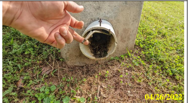
24. Toe drain at center of downstream dam face showing damaged animal guard
