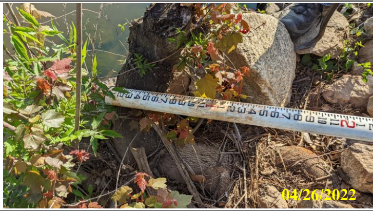
9. View of stump close to diameter requiring engineer oversight for removal, located on right side of upstream dam face at waterline
