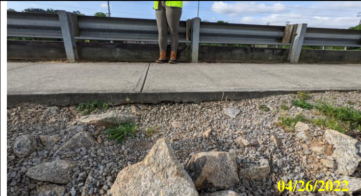
21. Minor undercutting and erosion at the pedestrian walkway on upstream dam crest
