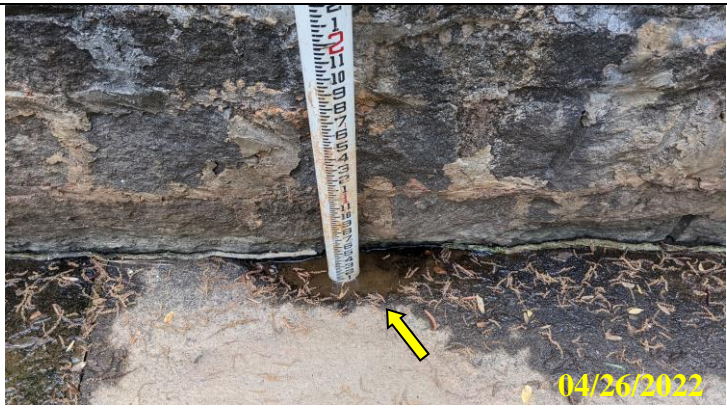
33. Concrete spillway cracking and missing concrete at masonry wall joint
