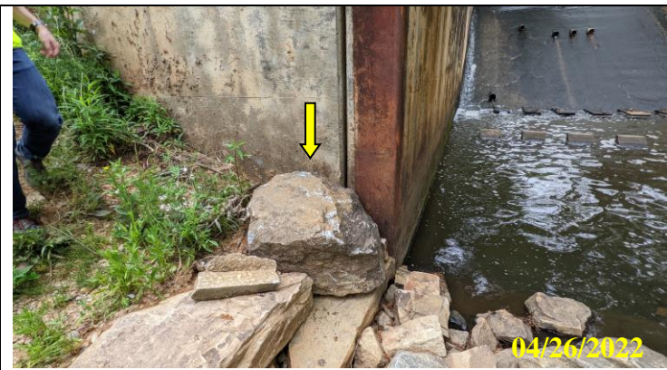
25. Toe drain at right side of plunge pool blocked by riprap
