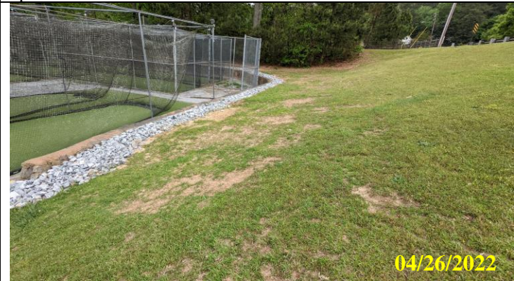
23. Right side of downstream dam face showing erosion and missing grass from equipment traffic
