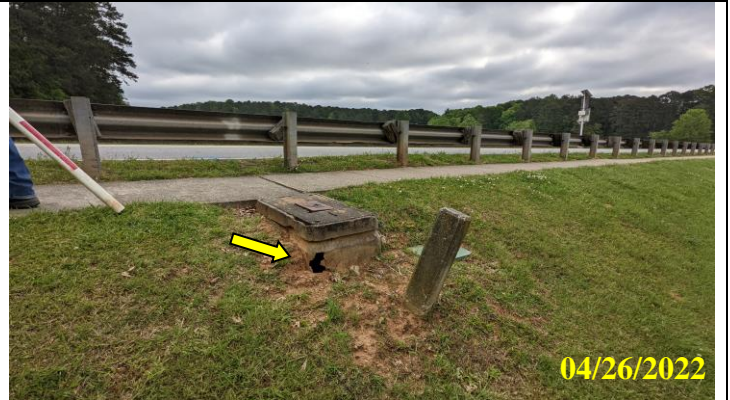
22. Damaged utility box and eroded soil on downstream face of dam
