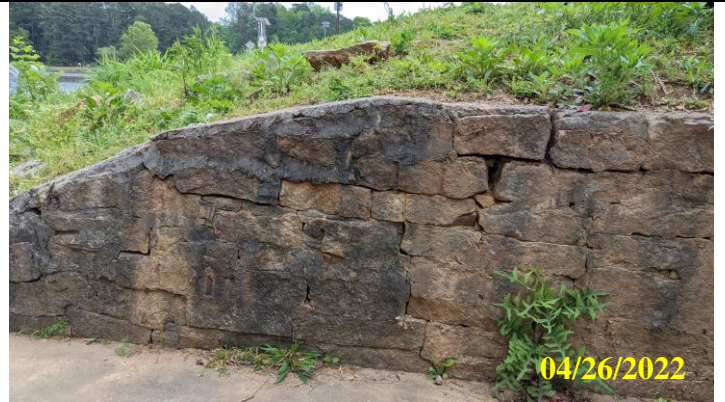
36. Missing grout and cracks in masonry wall at spillway entrance
