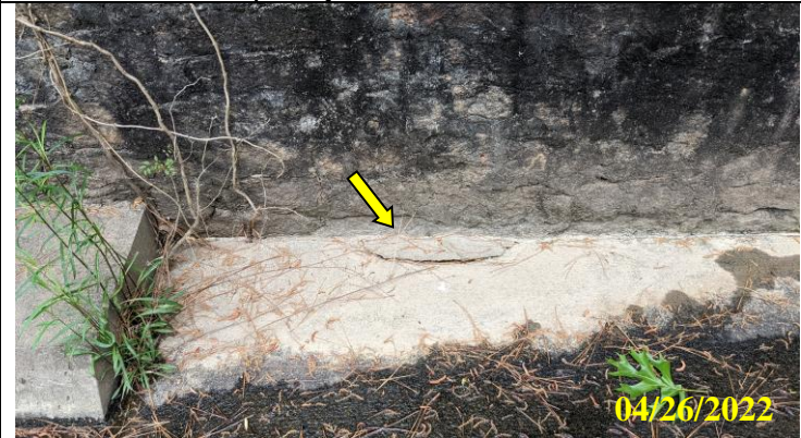
31. Concrete spillway cracking and uplift at joint with masonry wall
