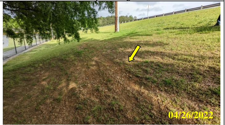
20. Patches of missing grass on downstream dam face
