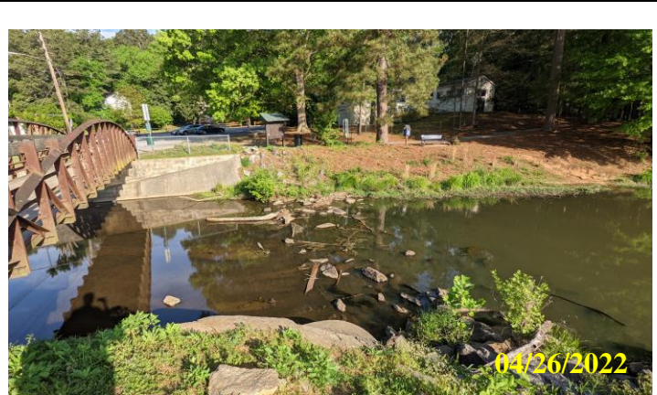
30. Cleared vegetation from right side of spillway, sparse riprap along the right wing wall
