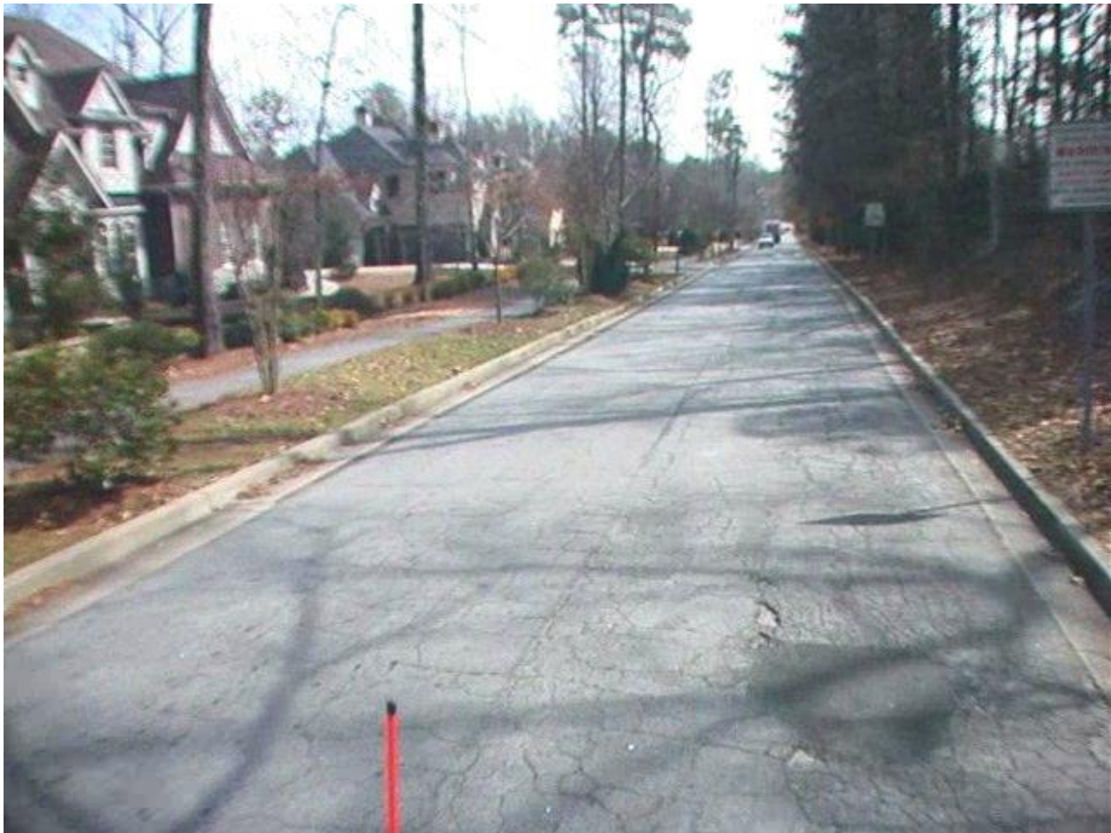
Brookhaven Drive, PCI = 41, This is the Worst Part of the Roadway
