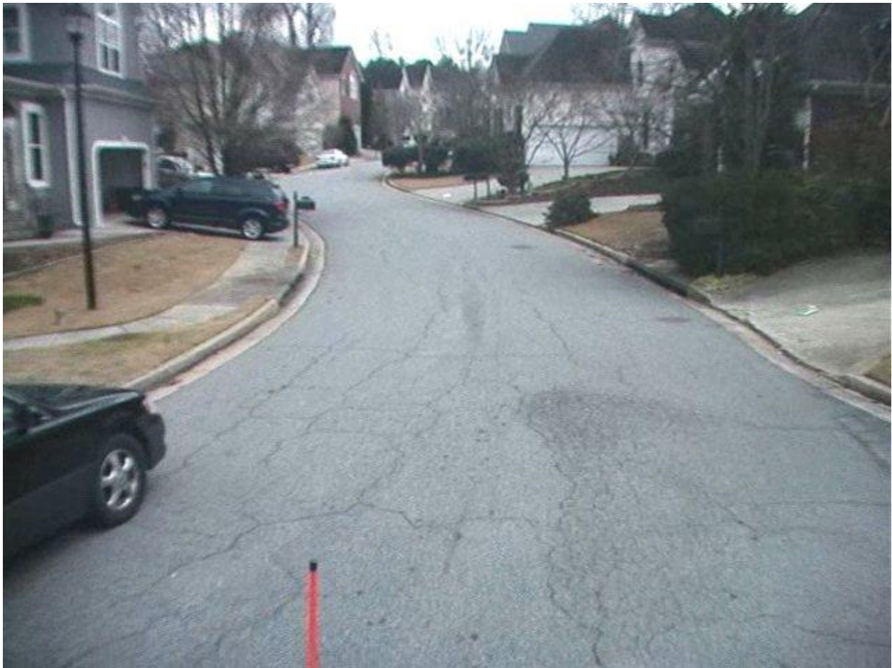
Wayside Dr, PCI = 55, Just Starting to Fail in Local Areas
