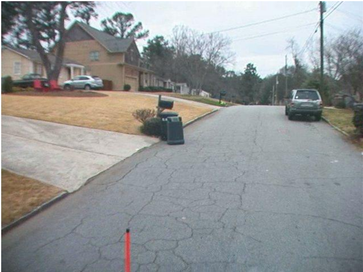
Ringle Road, PCI = 65, Just Starting to Show Non-Load Associated Cracking and Distresses That May be Repaired and Covered
