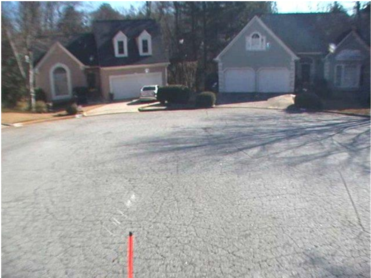
Bankshill Row, PCI = 12, The Entire Street Has Failed
