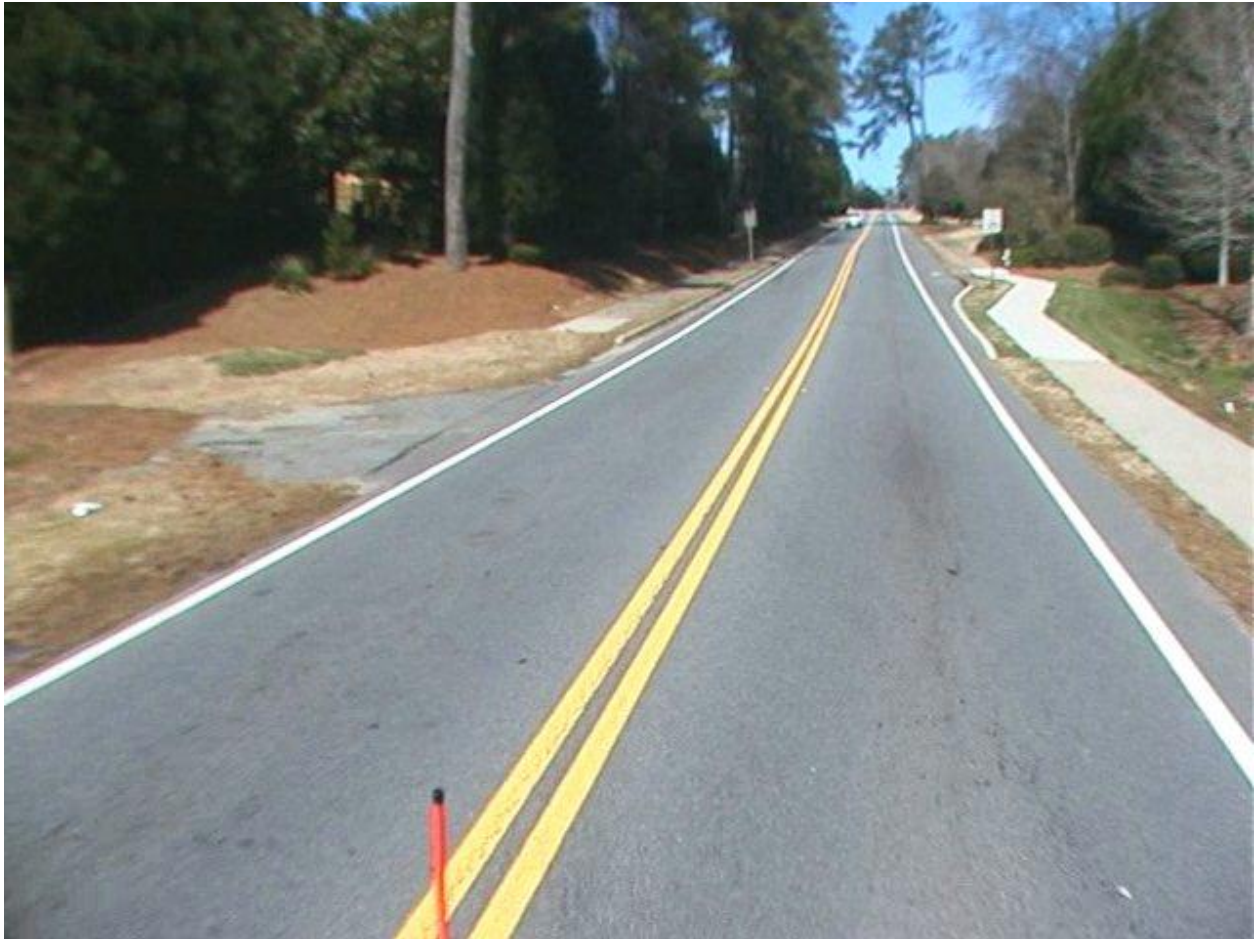
Johnson Ferry Road, PCI = 86 and the Surface is Distress Free, Smooth and Ready to Provide Years of Good Service
