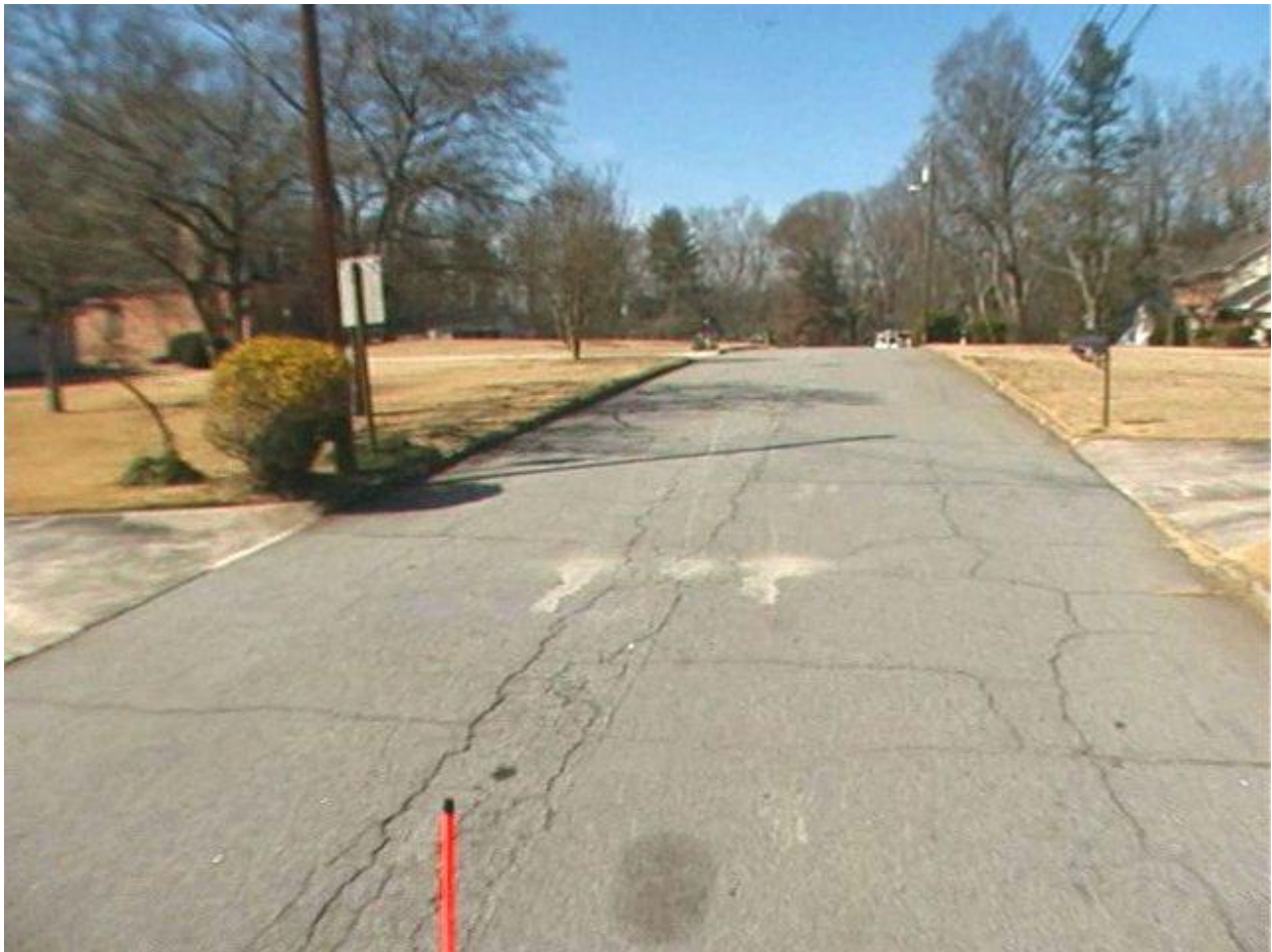
Parkcrest Drive, PCI = 45, Just Starting to Fail in Larger Areas and Become Rutted
