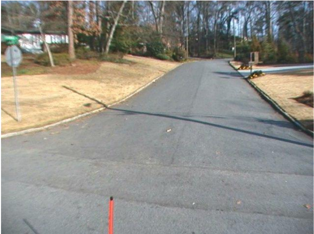
Shawnee Lane, PCI = 80, Performing Well With Only a Couple of Minor Cracks
