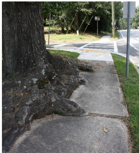
FIGURE 7. EXISTING SIDEWALK OBSTRUCTED BY TREE ROOTS NEAR CHILDERS ROAD OBSERVED DURING FIELD VISIT
