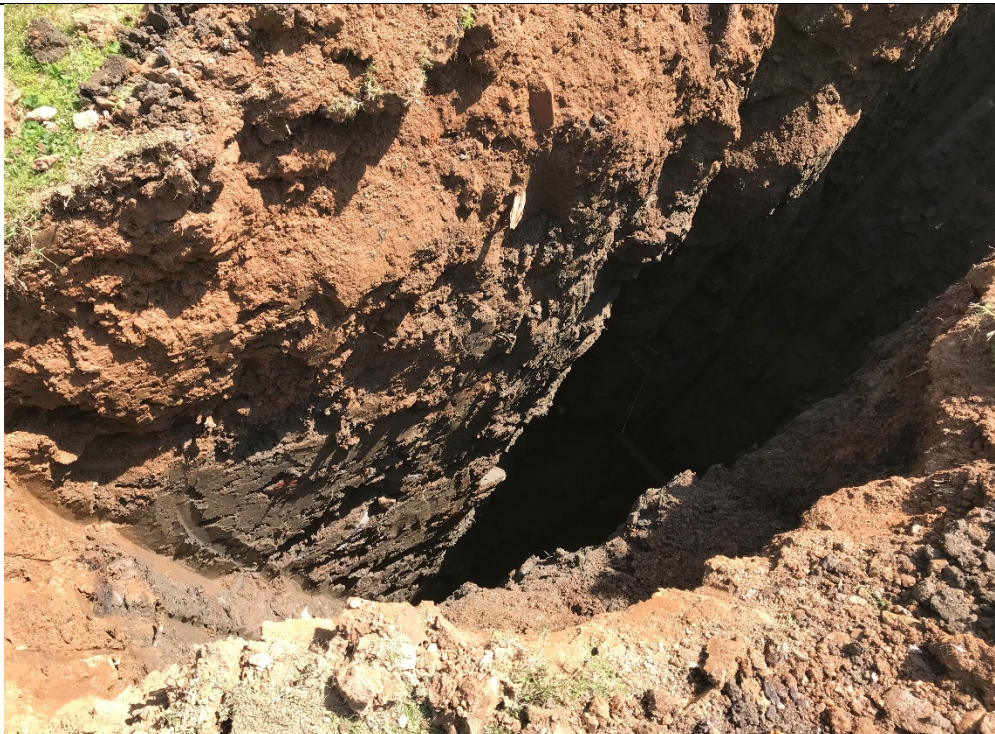
TP-1 - Approximately 2 feet of "clean" fill cover followed by debris-laden soil and organic refuse. No groundwater encountered.
