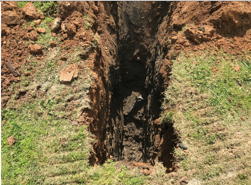
TP-2 - Approximately 3 feet of "clean" fill cover followed by debris-laden soil and organic refuse. No groundwater encountered.
