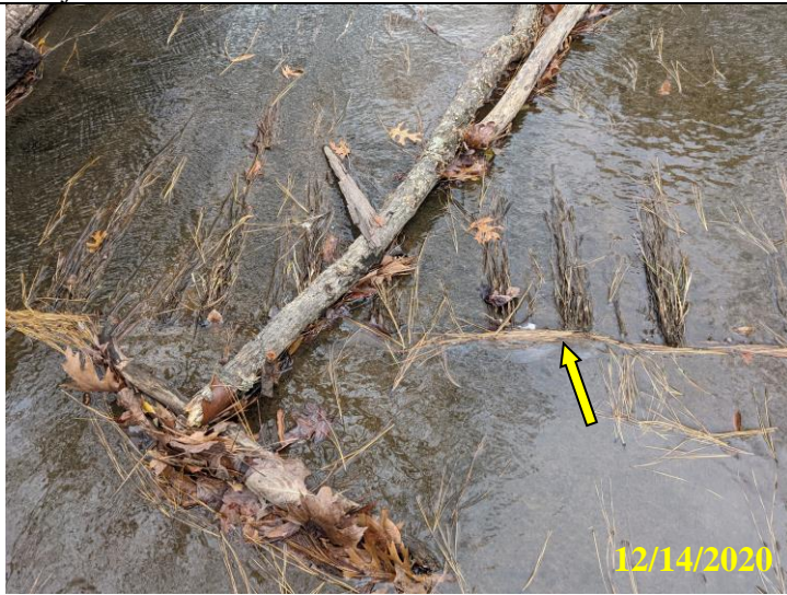
35. Grass growing between slabs in concrete spillway
