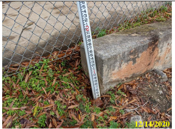
44. Minor undercutting and erosion at the end of the concrete spillway wall. See Photo 45 for location
