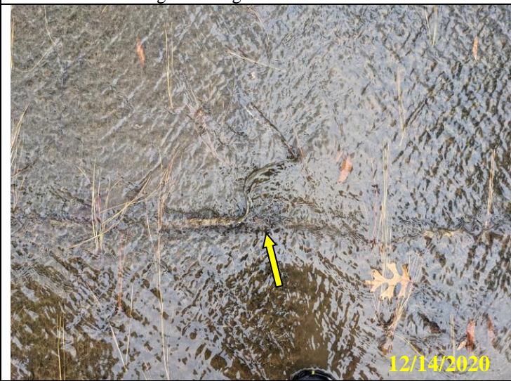
41. Caulk peeling from between spillway slabs downstream of bridge crossing
