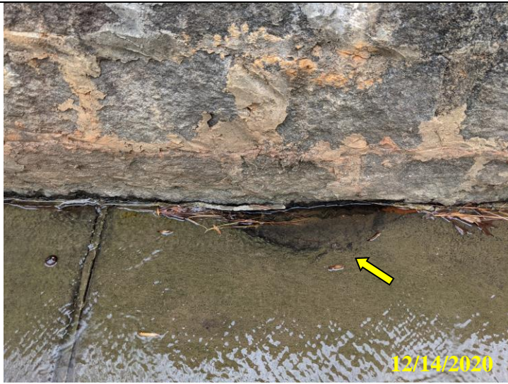
33. Concrete spillway cracking and spalling concrete at masonry wall joint
