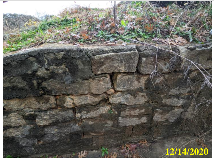
36. Missing grout and cracks in masonry wall at spillway entrance
