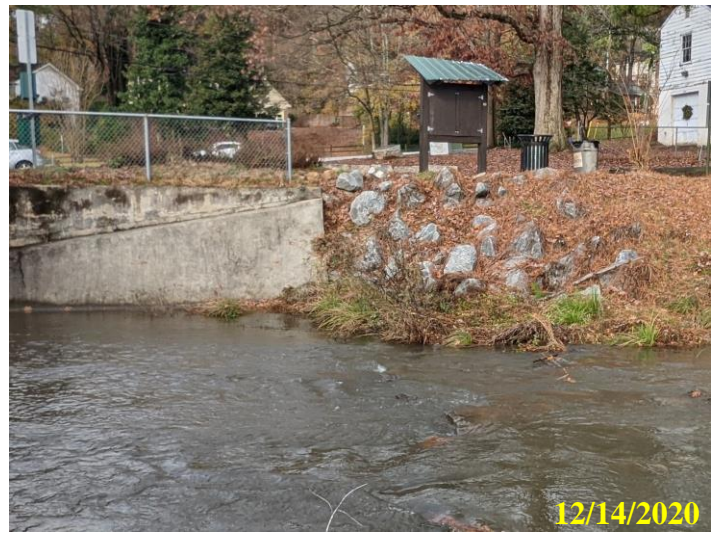
30. Vegetation and silt obstructing right side of upstream spillway. Sparse riprap along the right wing wall of the spillway
