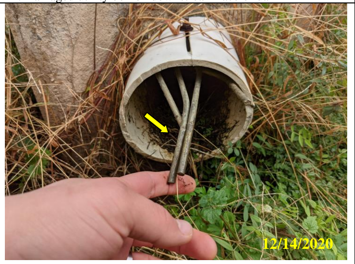
24. Toe drain at center of downstream dam face showing damaged animal guard.
