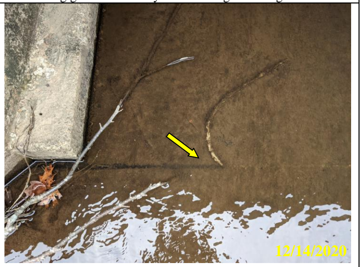
40. Caulking peeling from between spillway slabs at bridge crossing
