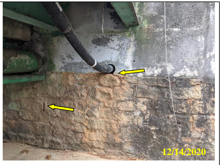
38. Missing grout in masonry wall at bridge crossing
