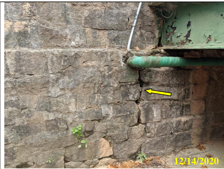
37. Missing grout in masonry wall at bridge crossing
