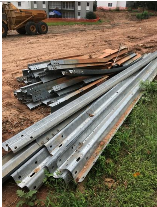
City furnished steel posts, w-beams, and spacer blocks to be installed in replaced section.
