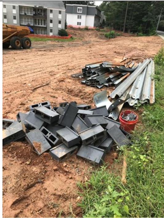
City furnished steel posts, w-beams, and spacer blocks to be installed in replaced section.
