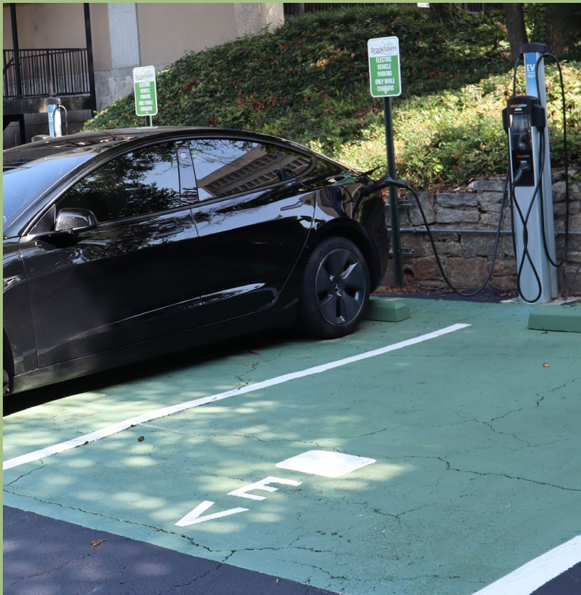
EV charging stations at Brookhaven City Hall
