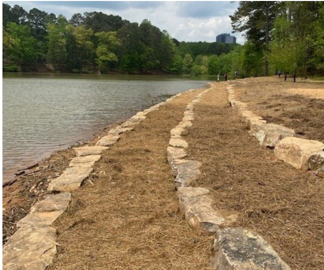
Brookhaven completed the shoreline restoration of the east banks of Murphey Candler Lake during the pandemic shutdown.
